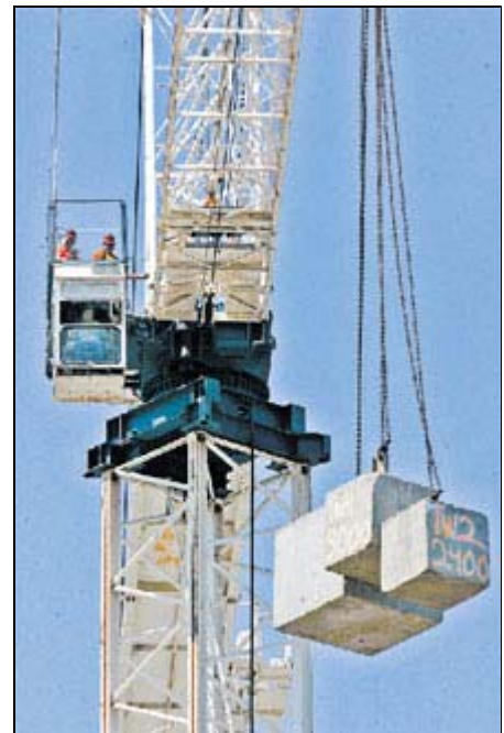
LAURA EMBRY / Union-Tribune Robert Jennings of the Tower Crane Task Force (left) and crane technician Matt Finnerty inspected a tower crane last week while Bobby Oulette of H.P. Forming International Inc. operated the crane and lifted thousands of pounds to test the jib.
